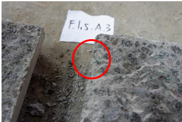
Figure 6. The Full-sized Length of Welded Wire Mesh Sticking Out from the Concrete Surface
