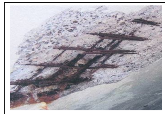
Gambar 2. Spalling selimut beton
