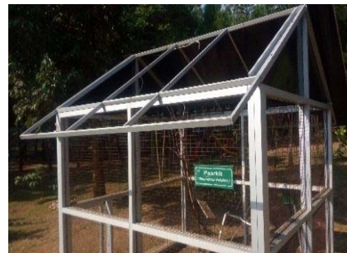
Figure 16. Roof on the bird cage damaged
