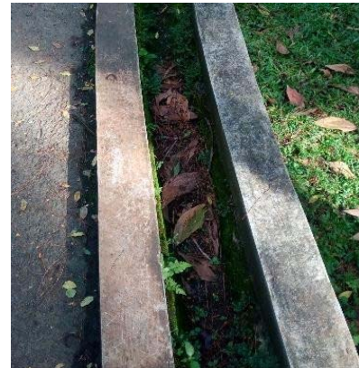
Figure 14. Garbage on the park gutter.
