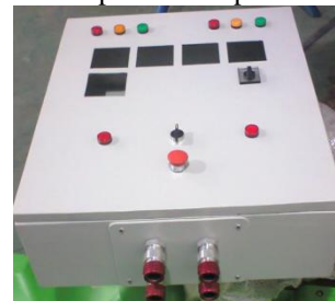
Gambar 31 Box Panel ATS/AMF
