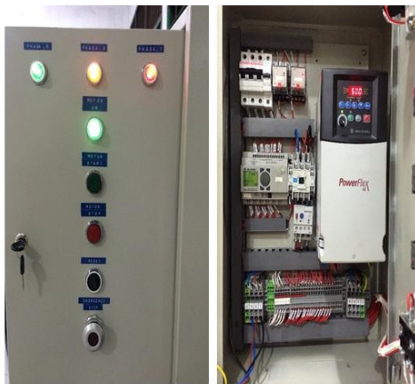
Gambar 5 Panel kontrol motor generator
