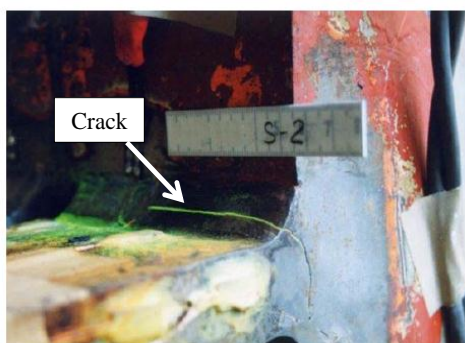
Figure 1. Fatigue Crack Occurred at Beam-to-Column Connection [1]
