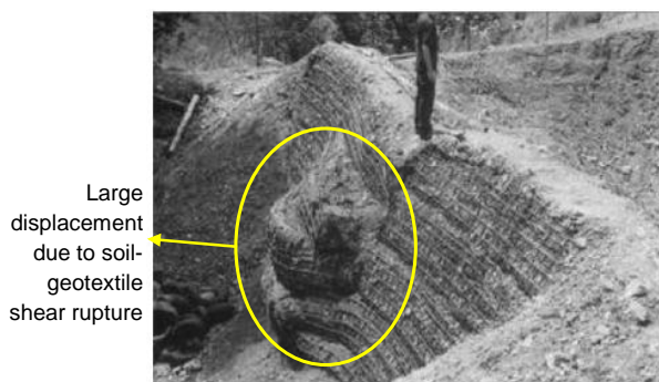
Figure 2. Reinforcement Layers Offer a Preferential Plane for Shear Rupture: Rockfall Protection Embankment [10]
