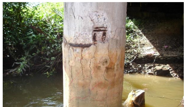
Figure 5a. Cracking, Delamination, and Spalling with Exposed Rebar on Column C1
