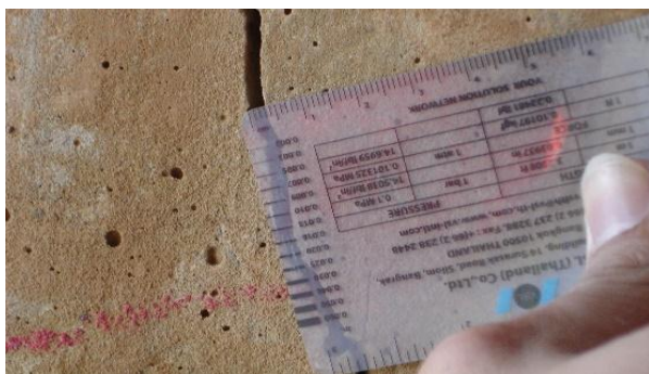
Figure 3. Three mm Crack Found on Column C1
