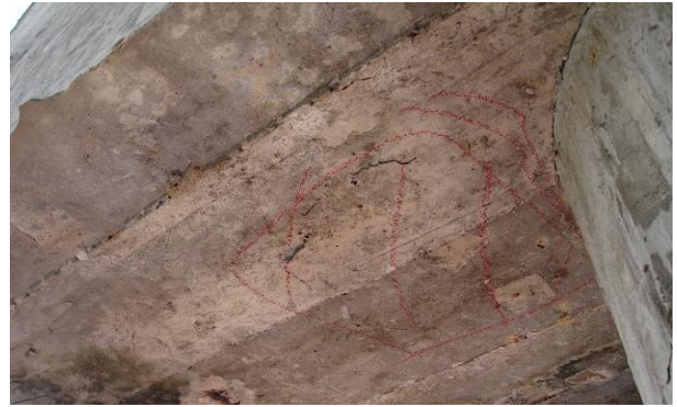
Figure 4b. Delamination Detected on Beam B1
