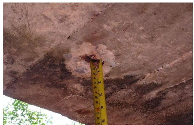
Figure 5c. Exposed Rebar with 10mm Cover on Beam B1 Soffit
