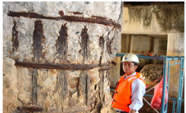
Figure 5b. Concrete Spalling Exposing Severely Corroded Rebars on Column C9
