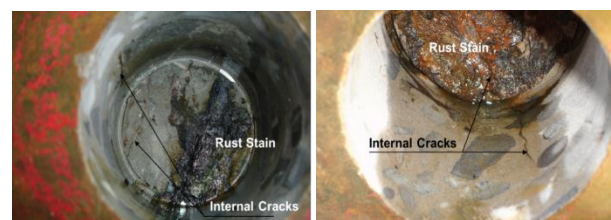
Figure 11. Rust Stain and Internal Cracks Found Inside the Core C-4 and Core C-3 in Location on Column C6 and Column C4, respectively.
