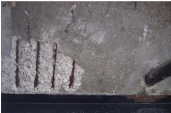
Figure 5d. Concrete Spalling with Exposed Corroded Rebars on Deck Soffit
