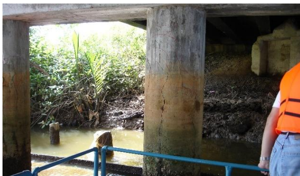
Figure 4a. Delamination Detected on Column C2
