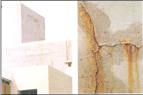
Figure 3. Cracking due to reinforcement corrosion [1]
