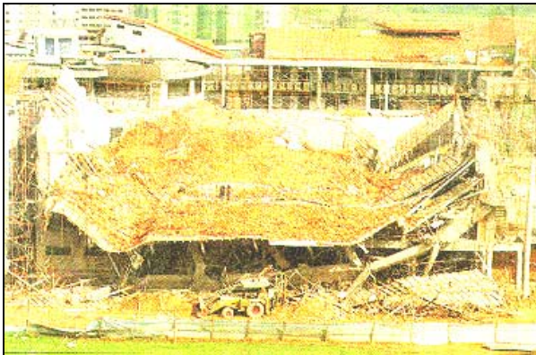
Figure 2. The roof collapse of Compassvale primary School's multipurpose hall (in June 1999) had caused 7 workers injured. It is due to bad welding work at roof steel joints.
