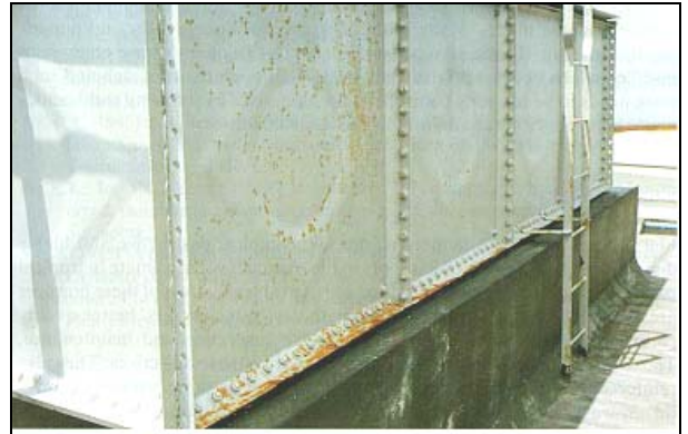
Figure 6. Water tank corrosion [3]
