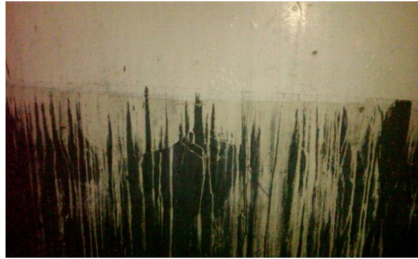
Figure 2. Showing Stains on Wall
