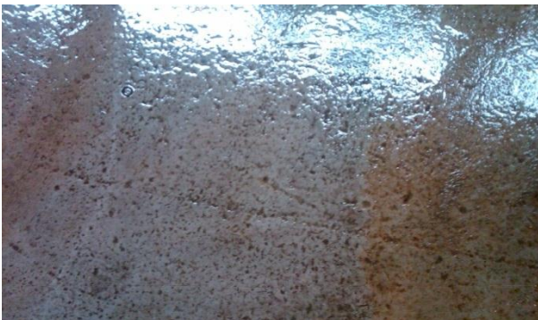
Figure 1. Wearing of Floor Finish due to Abrasion
