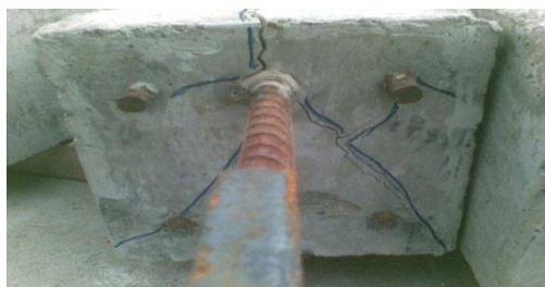
Figure 2(b). Failure of OPC Concrete Specimen
