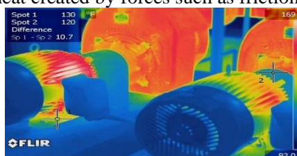
Figures 6. Thermocam Image Results on Electrical Machines
