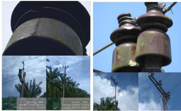
Figures 12. Material Replacement Based on Thermacam Inspection
