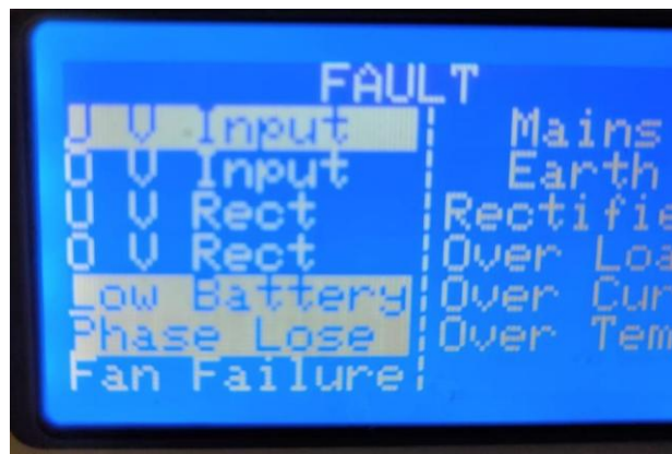
Figure 6. Rectifier Indication Display
