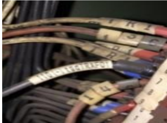
Figure 8. Cable Cause DC Ground
