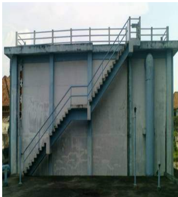
Gambar 8. Bak Reservoir Booster U.P KM4
