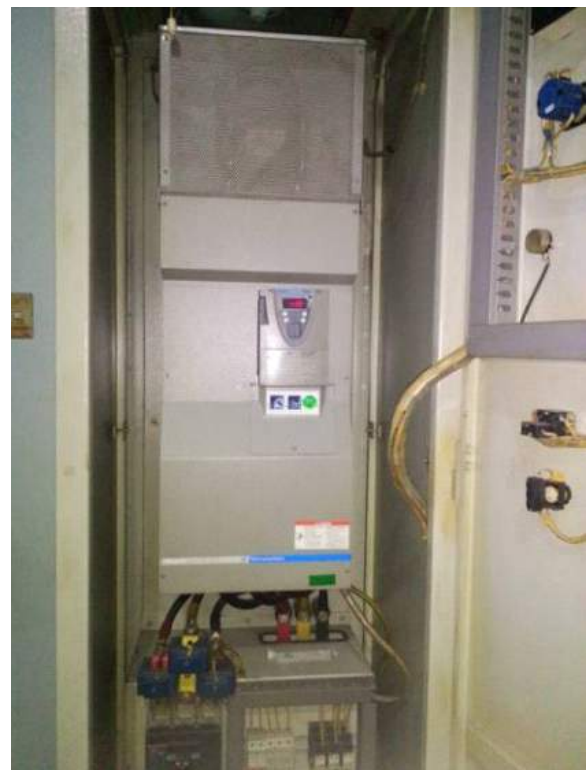
Gambar 17. Panel Inverter di PDAM Tirta Musi Unit Pelayanan KM IV Palembang
