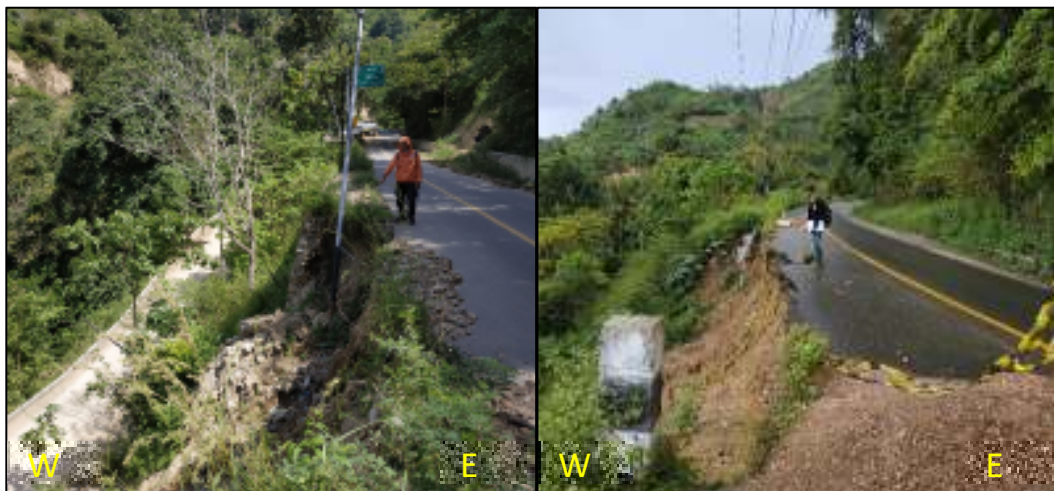
Figure 20. Landslide Incident in Olele Village
