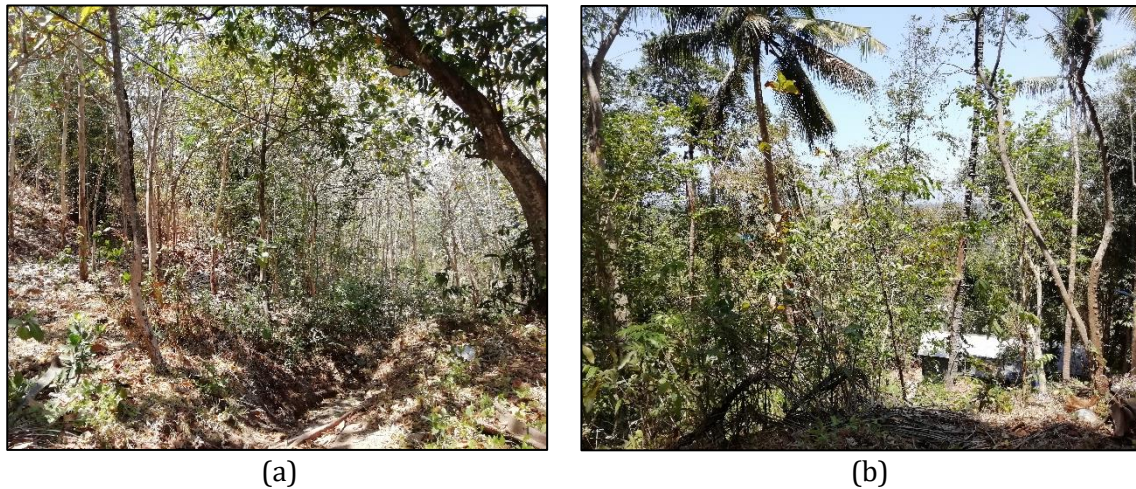
Figure 2. Conditions hill in Kretek, Parangtritis, 2019. a) Erosion damage due to the flow of rainwater b) Foot slope, which uses as a place of settlement very range of landslide hazards. (Source: Field observations, 2019)
