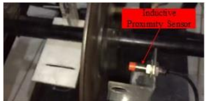
Figure 9. Instalasi And Location Of The Inductive Proximity Sensor
