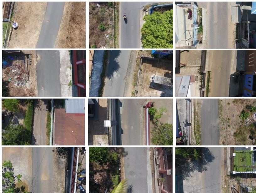
Figure 2. Pothole capture from each video data
