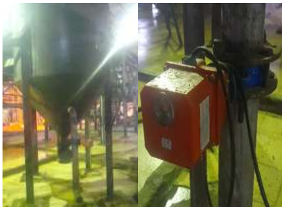
Gambar 10. Automatic Valve Drain Sand Trap Tank Jenis Electric Valve
