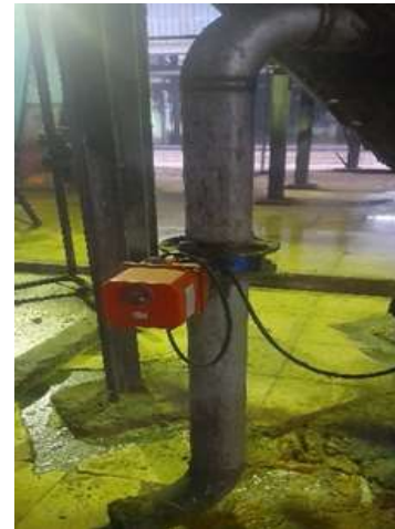
Gambar 11. Automatic Valve Drain Sand Trap Tank Jenis Electric Valve
