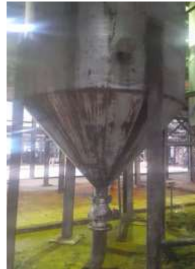
Gambar 5. Sand Trap Tank Pabrik Kelapa Sawit
