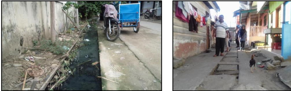
Figure 3. Drainage condition at four hamlets (Source: Observation)
