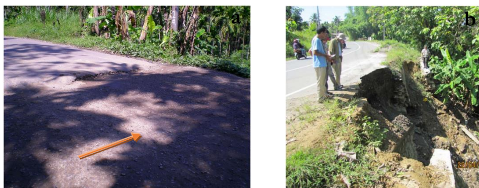
Figure 3. (a) Swelling clay cause soil creeping on the road, and (b) Swelling clay destroy the retaining wall in the Juli Sub – District
