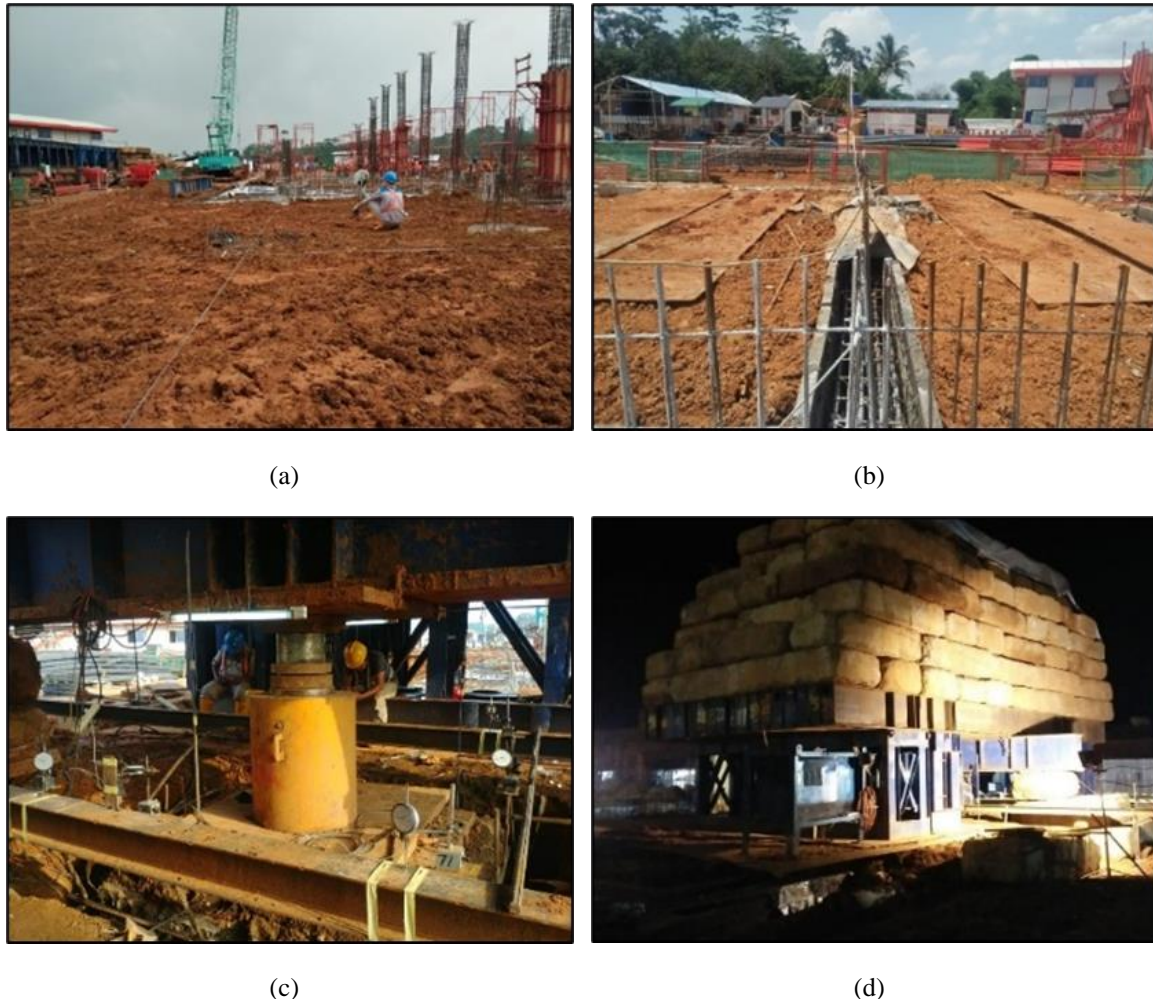
Figure 13 Kentledge preparation work: (a) Compaction of subgrade soil, (b) Steel plate placing, (c) Installation of kentledge footing, main beam, secondary beam, and concrete block, (d) Kentledge system during pile test.
