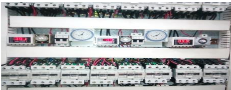
Figure 5. Optimization of the operating time of engine rooms and equipment of buildings, University of Kashan
