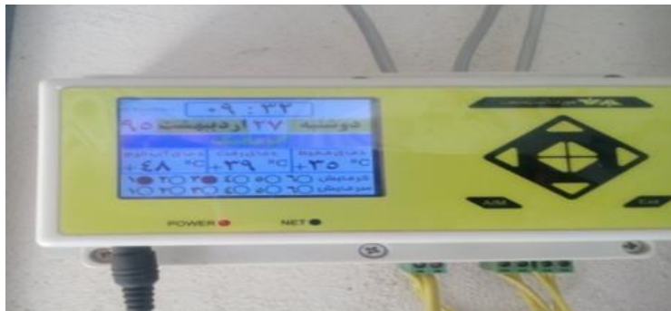
Figure 4. Intelligent control of the engine room (This system controls the volume of the burners by getting indoor and outdoor temperatures), University of Kashan, Iran
