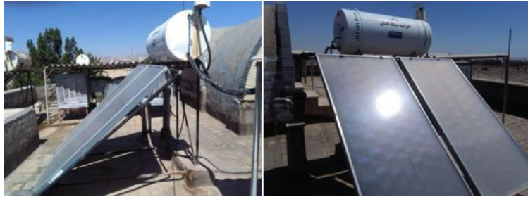
Figure 3. Installation of solar water heater for the supply of heated water for 14 buildings at University of Kashan, main campus.
