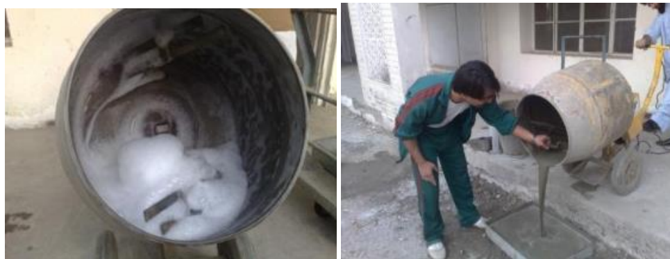
Figure 3. (a) Lightweight formation in mixer machine (b) Mortar foam
