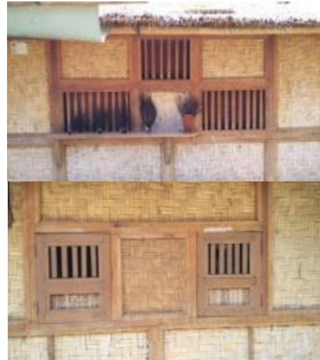
Figure 8. Several types of windows from wood materials in Bale Tani , in similar design Source: Author, 2017
