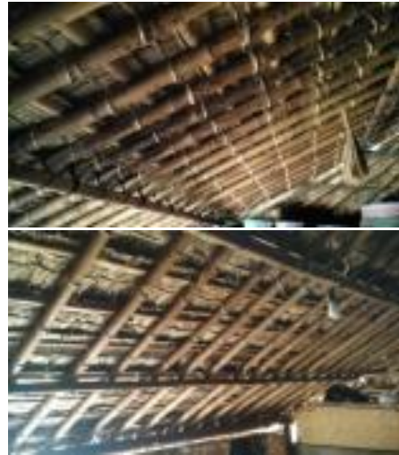
Figure 6. Top: Using a natural string, Bottom: Using a Nylon Rope Source: Author, 2017
