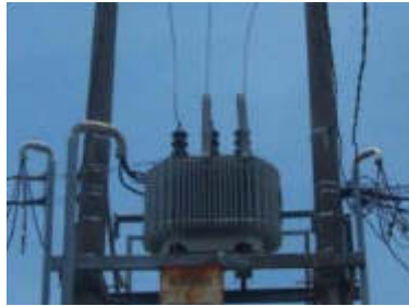
Image 1 Pole Transformer Pole
