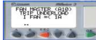
Gambar. 4.8 Tampilan trip fan A10 underload
