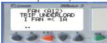
Gambar. 4.12 Tampilan trip fan A12 underload.
