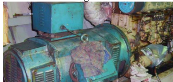
Figure 1. Engine Generator set owned by KM. Okishin 07
