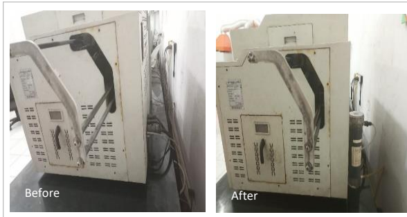
Fig. 6. Improvement with UPS installation
