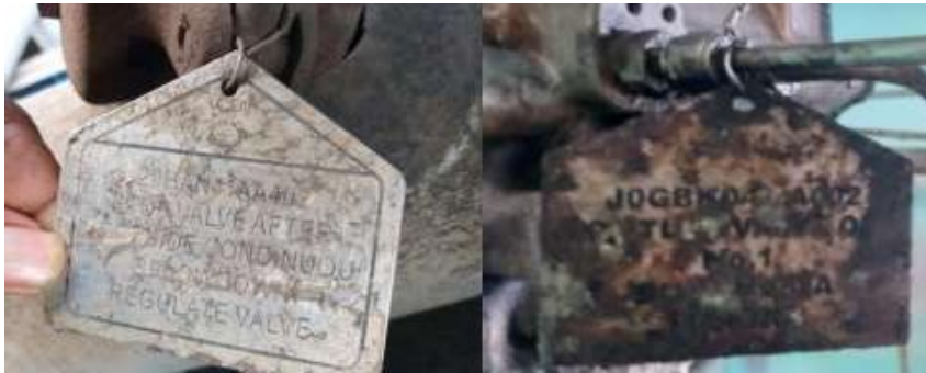
Figure 9. Corroded equipment nameplate
