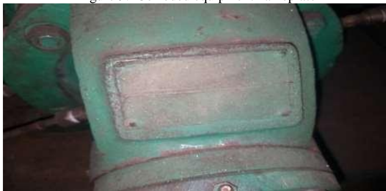
Figure 10. Equipment lost nameplate specification
