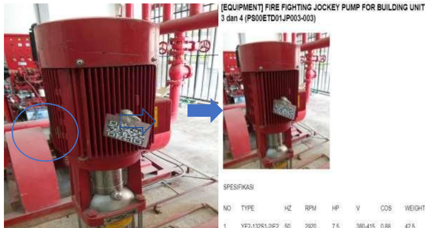
Figure 12. Utilizing qr code and scanning out results on equipment jockey pump
