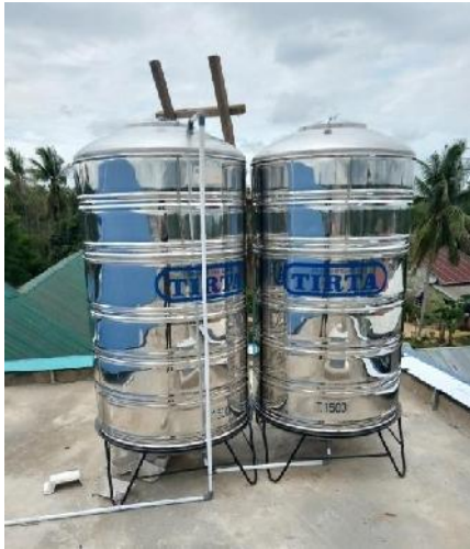
Gambar 3. Roof Tank / Recervoir
