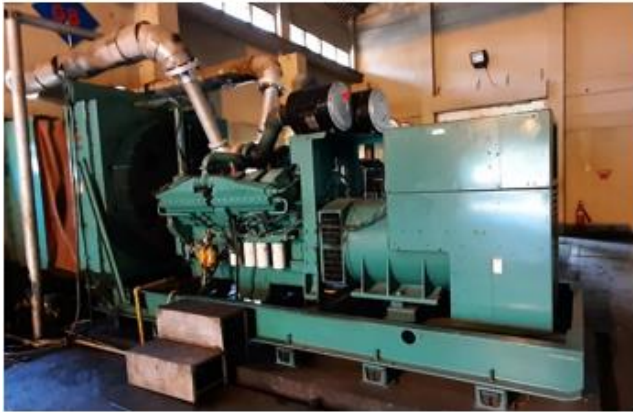
Figure 1 Generator Set 8 in the PPSDM Migas power plant unit
