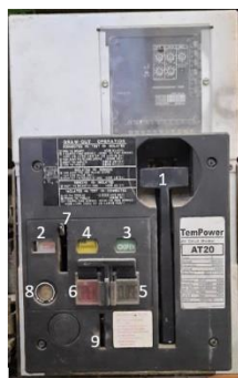
Figure 2 Air Circuit Breaker (ACB) Genset 8 in the Power Plant Unit they are part of a sentence, as in
