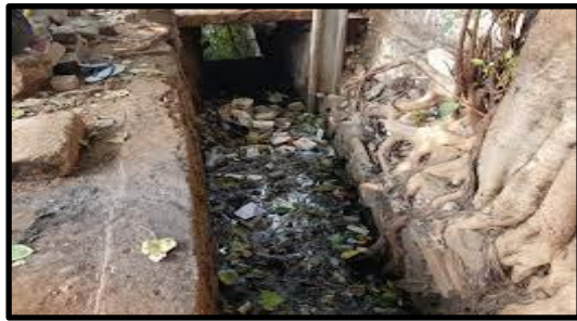
Figure 3 Drainage Damage and Garbage (Sumber: Palpos, 2/12/2019, Kec. Sukarami Palembang)
