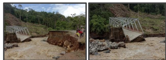
Figure 1. Damage to Mulak Ulu Bridge Construction (Link in Lahat and Muara Enim Regencies, South Sumatra). (Sumber: BPBD Sumsel, 30 Desember 2019)
