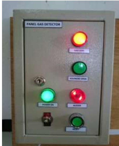
Gambar 9. Panel Gas Detector
