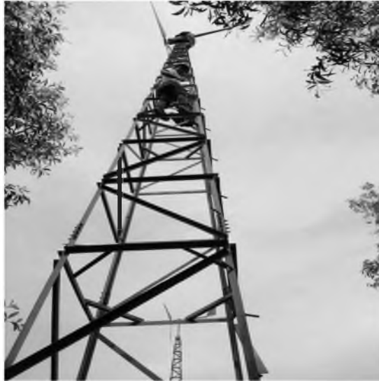
Gambar 2. Pengecekan Turbin Angin On site
