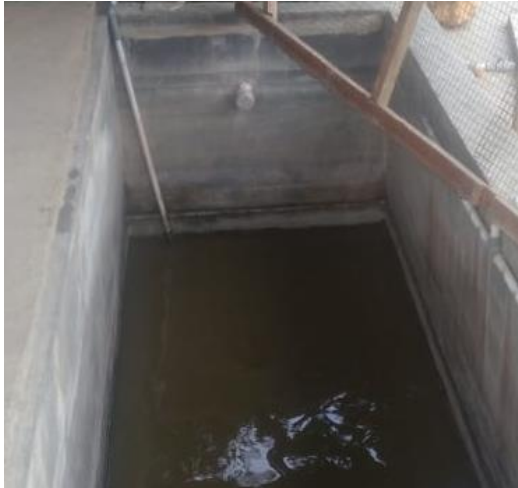
Gambar 3. Bak kontrol effluent IPAL
