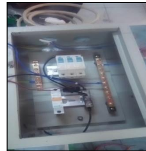
Gambar 7. Box Control Panel
