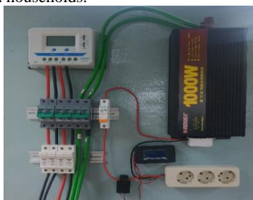
Fig 13. Off-Grid System Device
