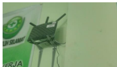
Figure 2. The first AP position in East Lab 2
