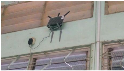
Figure 5. The first AP position in East Lab 2
