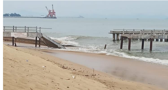
Fig 1. Damage of The Flying Bridge Due to The Impact of Pasir Panjang Beach Abrasion
