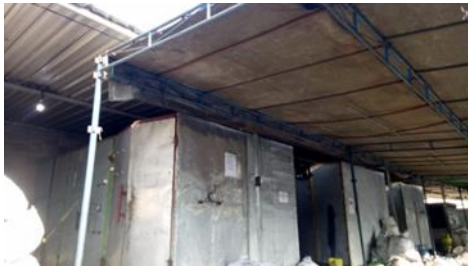
Figure 5 The briquettes Semi-permanent oven
