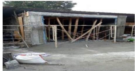
Figure 6 New permanent oven, size 4x3x2,5 m (still in the development stage)
