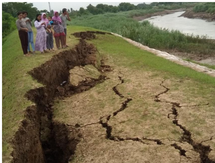
Figure 7. River embankment failure (Source: http://www.rmoljabar.com/read/2017/12/27 )
