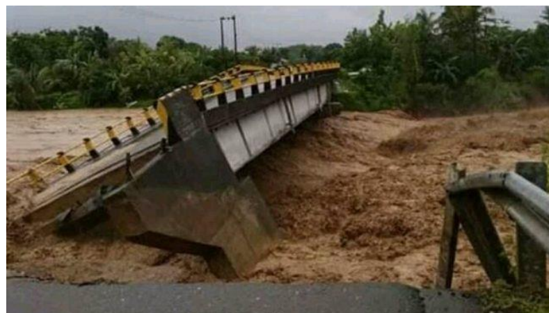
Figure 10. Bridge failure at Gowa, Sulawesi (Source: http://news.djournalist.com/read/2019/ )
