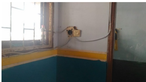
Gambar 4. Stop Kontak Laboratorium
