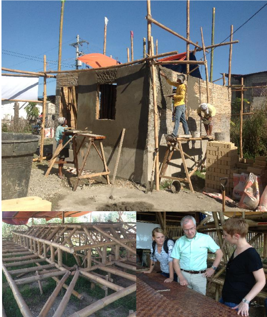
Figure 10. First Bamboo Demonstration House in Iloilo, Philippines, Bamboo Roof Structure, Pressed Bamboo Panels
