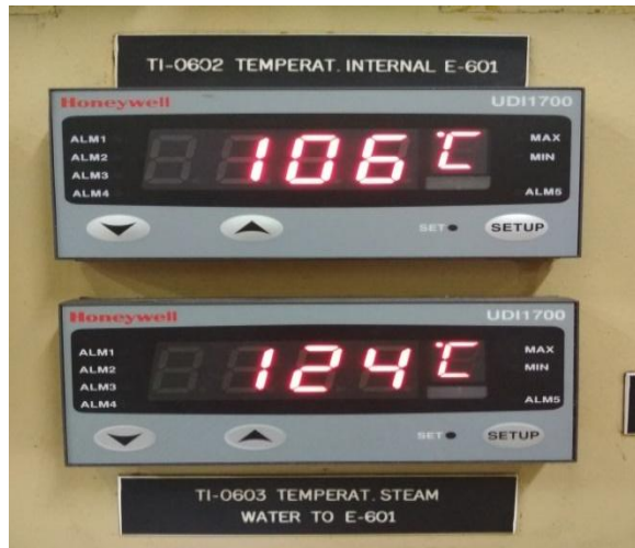
Gambar 3. Panel Kontrol suhu steam dan suhu didalam evaporator E-601
