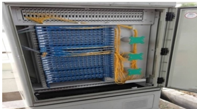
Figure 4: Optical Distribution Cabinet
