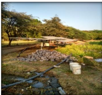
Figure 3. Solar water pumping system of study area
