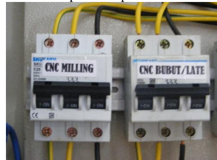
Gambar 3. Main Switch Posisi ON
