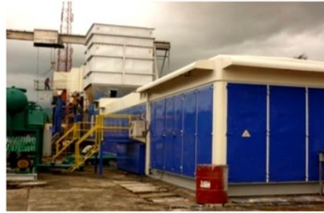
Figure 2 Gas Turbine PG 5341
