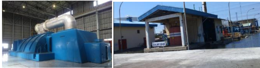
Gambar 2. Turbin uap dan auxiliary boiler .
